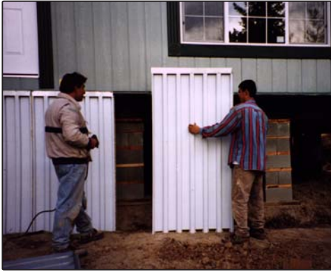
Panels attach around the perimeter of a soft-set. They hang with the bottoms at the middle of a footing trench.
