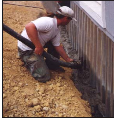
Just add concrete to the trenches, and the panel becomes a permanent foundation.
