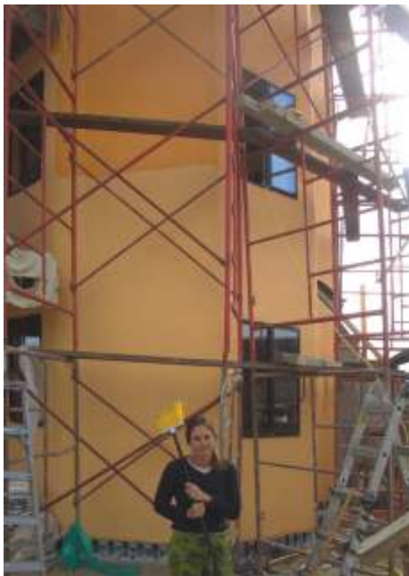
Plaster going over the panels - on a 3-story home in a 140 mph wind zone.
